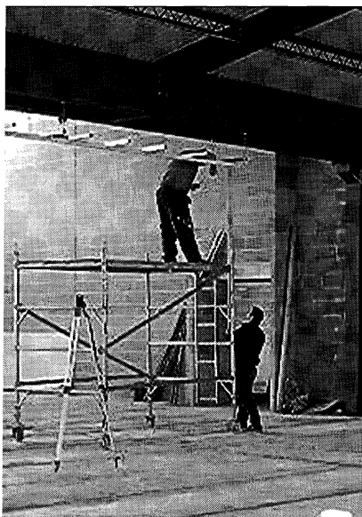
Pictured above is Byng Hall TTC's new premises under construction, at the St. John's Church of England Primary School in Tunbridge Wells
